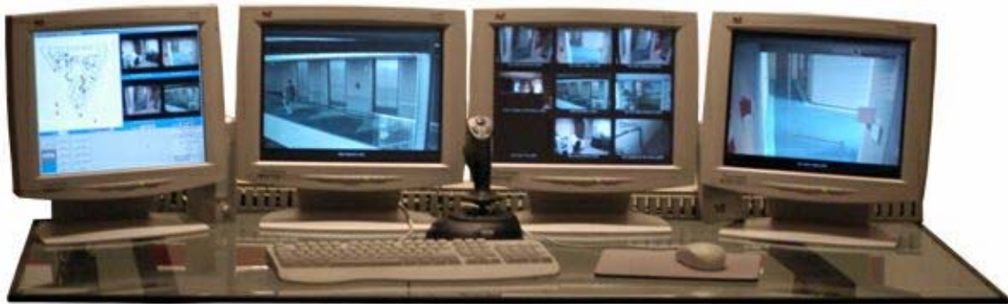
Figure 1-1. Typical Monitor Station
