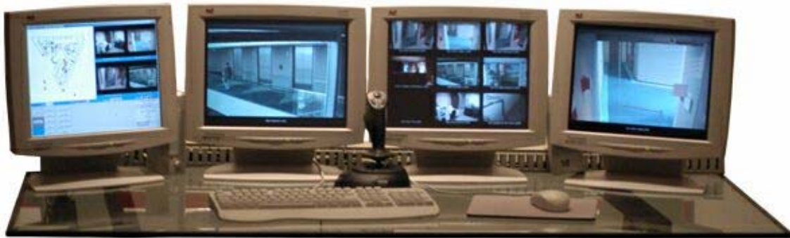
Figure 1-1. Typical Monitor Station
