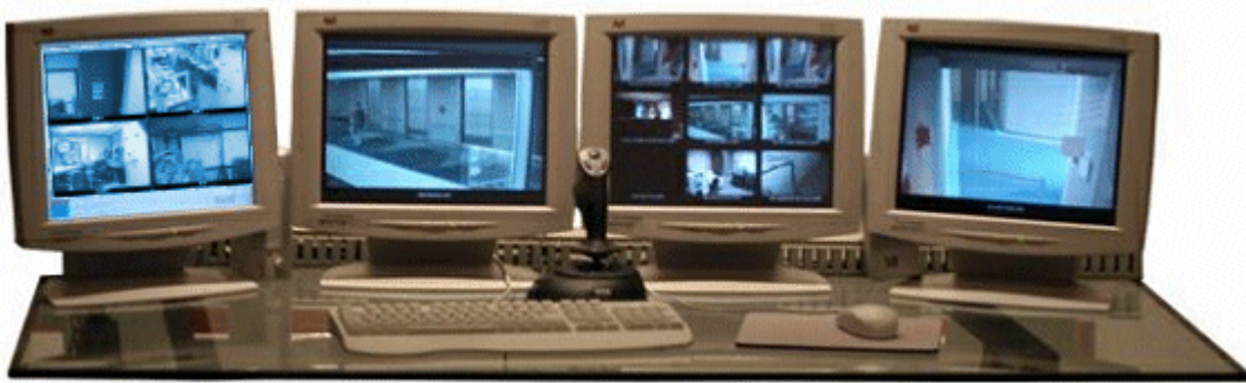
Figure 1-1. Typical Monitor Station
