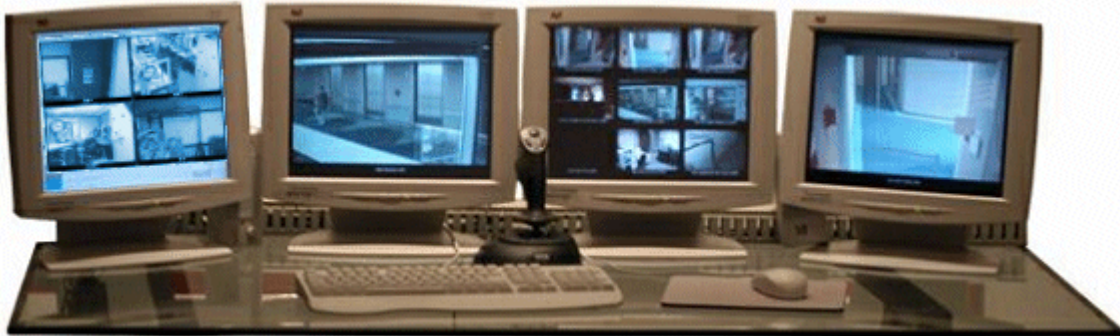
Figure 1-1. Typical Monitor Station
